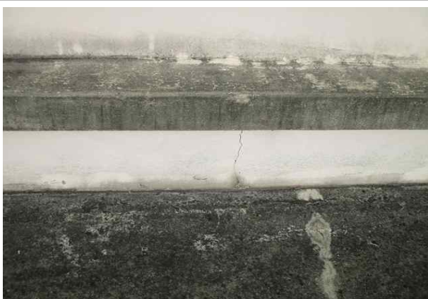
옥상층 벽체 균열 (CW=0.3mm, L=0.3m, 2EA)
