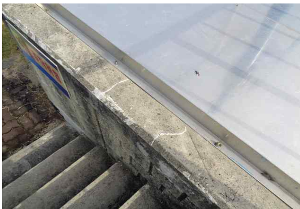
외부 벽체, 균열 (CW=0.1mm, L=0.5m, 2EA)
