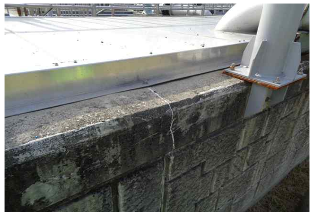
외부 벽체, 균열 (CW=0.1mm, L=1.0m)
